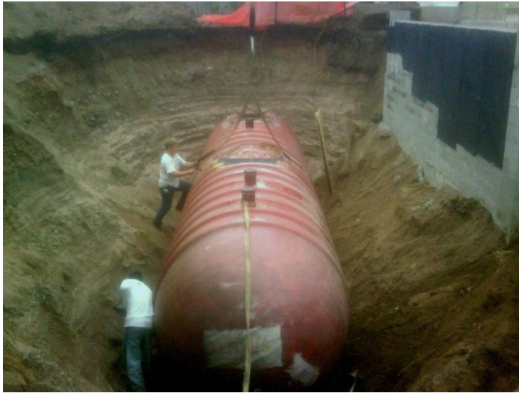
This 10,000 gallon storage tank was recently installed at one of our projects in St. Paul. Rainwater is captured from the site, held in the storage tank, then reused for irrigation purposes
